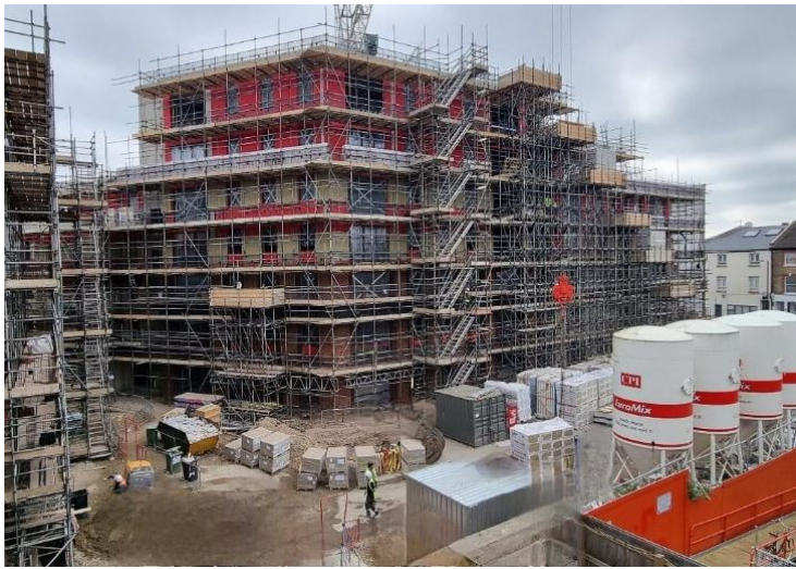
Block A/B (Right) and Block C (Left) image taken from top of Block C
