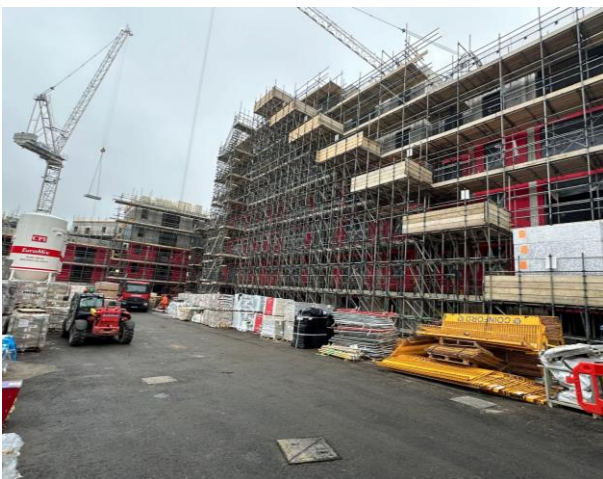
Block A (Right) and Block C1 (Background) from the Dawes Road site entrance
