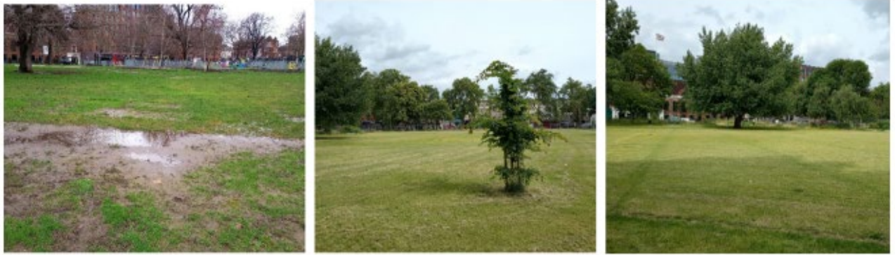
Figure 24: Shepherds Bush Green - Drainage works. Installed new land drains to the western field, which has been affected by surface water flooding during the winter months. The new system included underground drains, levelling the ground surface and grass seeding.
