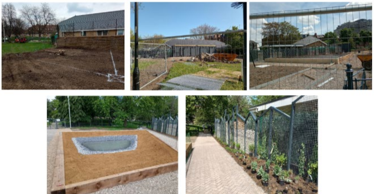
Figure 23: Frank Banfield Park - Construction of a new Community Garden and growing area, including landscaping, wildlife pond, raised beds, small orchard and containers.
