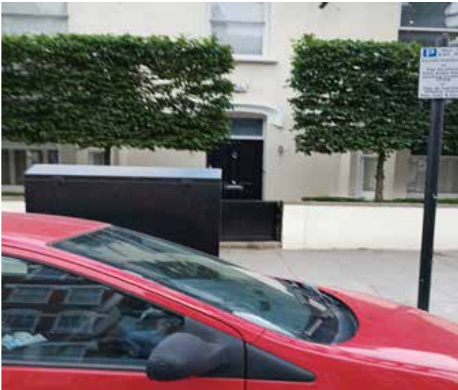
[Would you want this large utility cabinet outside the front door of your house?]
