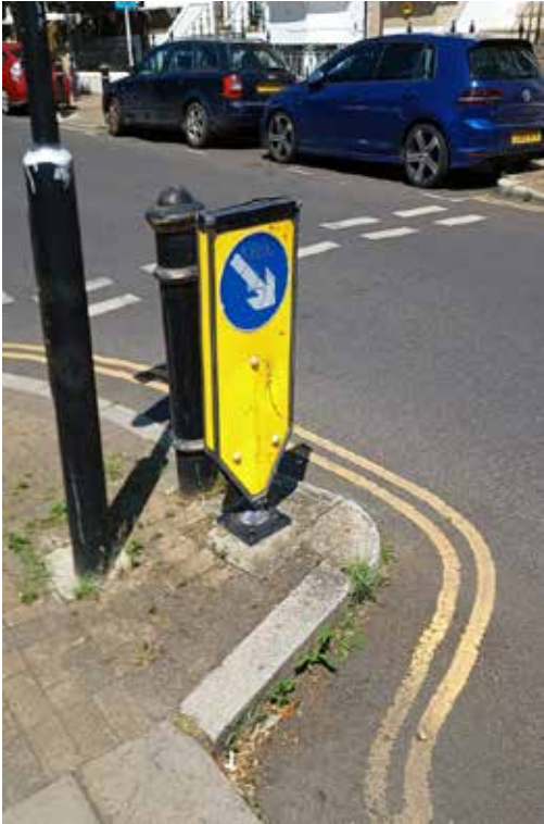
[Sulgrave Road – superfluous sign]
